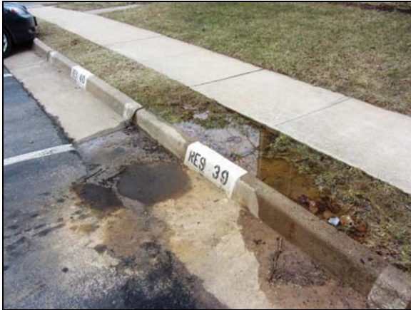
Photo #25. Defective grading between sidewalk and curb & gutter, Silverstone Court.
