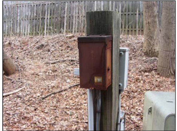
Photo #20. Common electrical service.
