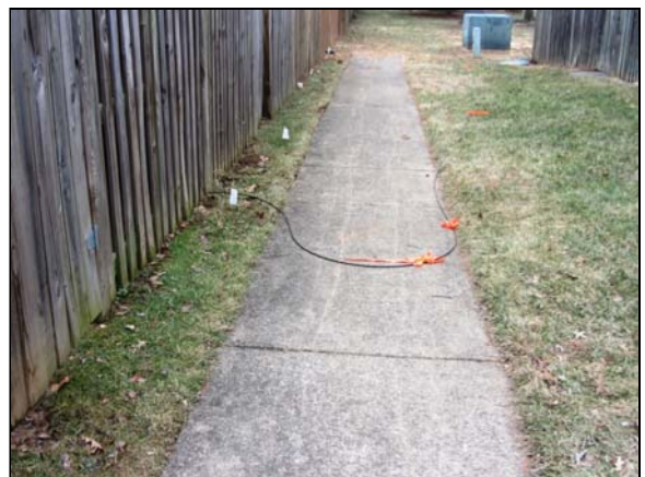
Photo #18. Utility companies have loose-laid wiring on sidewalk, Granite Creek Lane.
