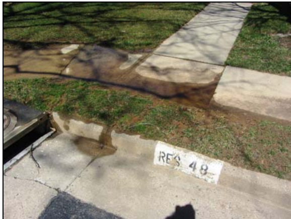
Photo #55. Defective grading and displaced sidewalk segments impound water and silt on the pavement, typical.
