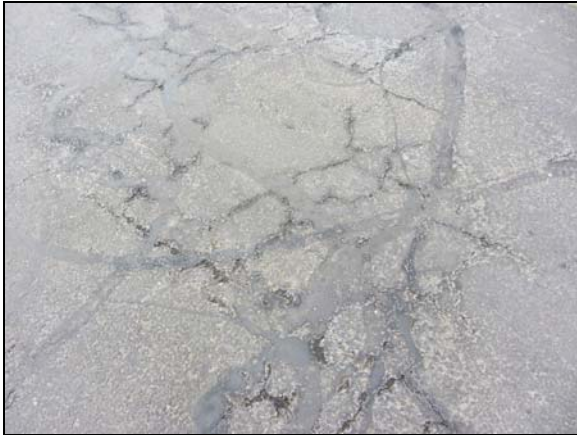
Photo #7. Typical alligatored asphalt pavement, Granite Creek Lane.
