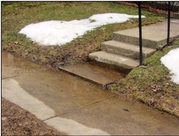
Photo #15. Height differences between sidewalks and lead walks are assumed to be the responsibility of the individual unit owners.
