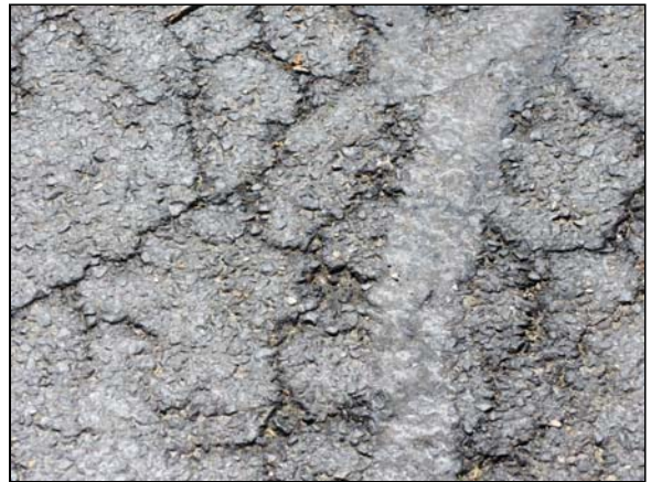
Photo #52. Typical deteriorated and alligatored asphalt pavement.
