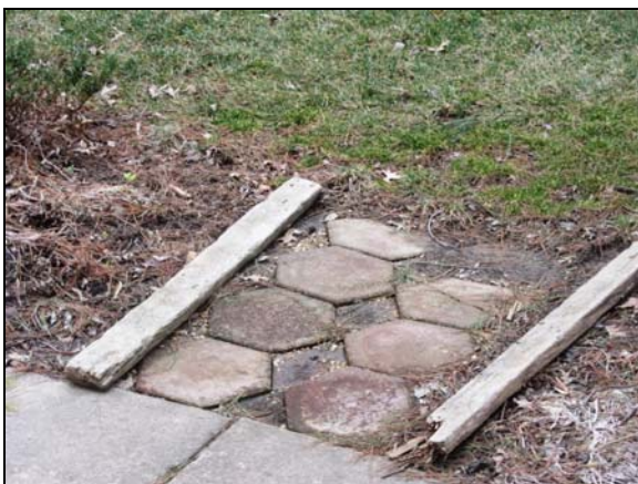
Photo #29. Limited paver installation at Silverstone Court leads to open space surrounding the stormwater impound facility.
