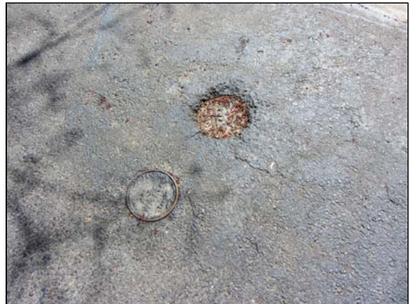
Photo #56. Defective utility access point impounds water, Granite Creek Lane.
