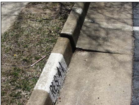
Photo #53. Displaced curb & gutter, typical.
