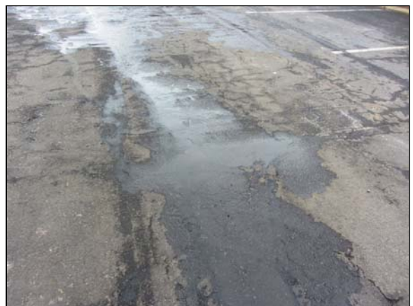
Photo #12. Standing water on asphalt pavement, Granite Creek Lane.
