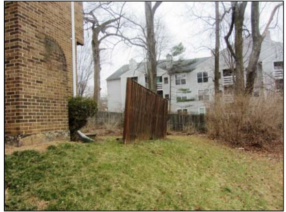
Photo #22. Limited wood fence installations at end unit, Granite Creek Lane
