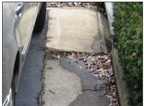
Photo #36. Displaced curb & gutter at stormwater inlet, Graystone Court.
