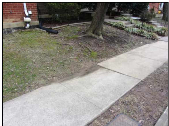
Photo #6. Displaced sidewalk and defective grading impounds water and silt on the concrete pavement, Granite Creek Lane.
