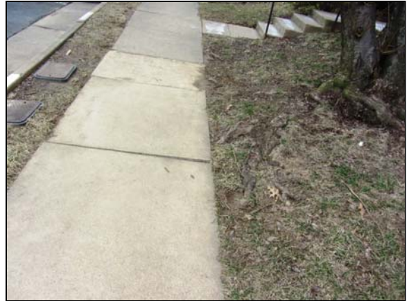
Photo #8. Defective grading between sidewalk and curb & gutter impounds water. Note displaced sidewalk, Granite Creek Lane.
