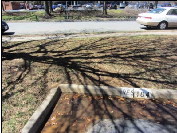
Photo #43. Typical depressed pavement and concrete curb & gutter may indicate damage to base materials and bearing soils beneath the asphalt pavement.
