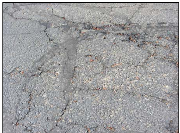
Photo #48. Typical alligatored asphalt pavement.
