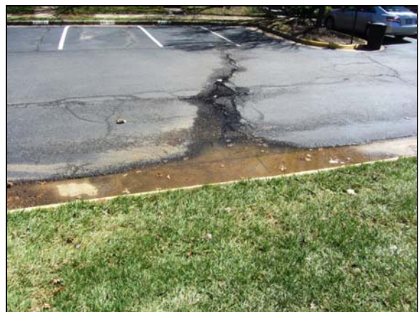
Photo #42. Typical depressed pavement and concrete curb & gutter may indicate damage to base materials and bearing soils beneath the asphalt pavement.
