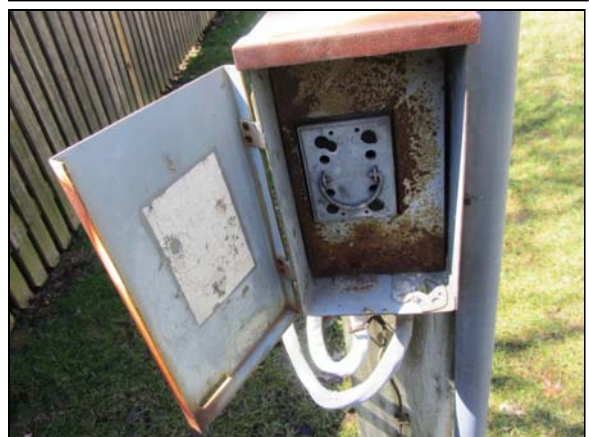
Photo #60. Detailed view of the electrical service between Graystone Court and Silverstone Court.
