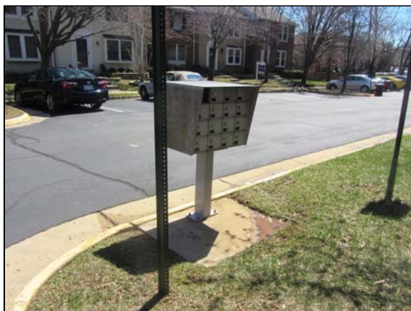
Photo #41. Start of photographs taken on March 31, 2014. Mailbox installation, Graystone Court. Note missing box door.
