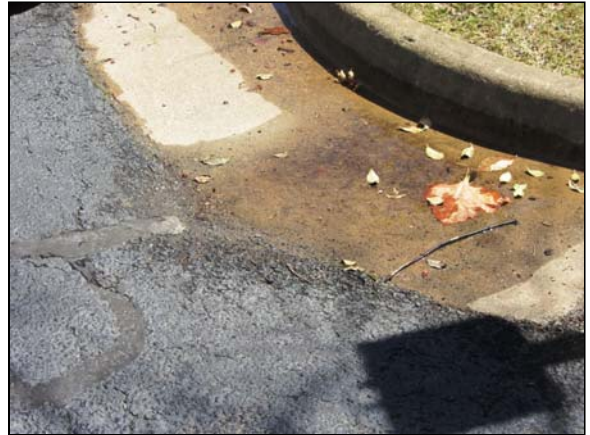
Photo #50. Typical depressed pavement and concrete curb & gutter may indicate damage to base materials and bearing soils beneath the asphalt pavement.
