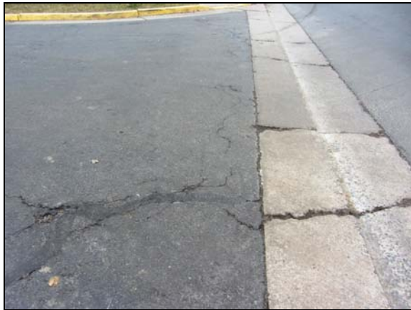
Photo #3. Asphalt pavement and concrete apron at the intersection of Granite Creek Lane and Flagpole Lane.
