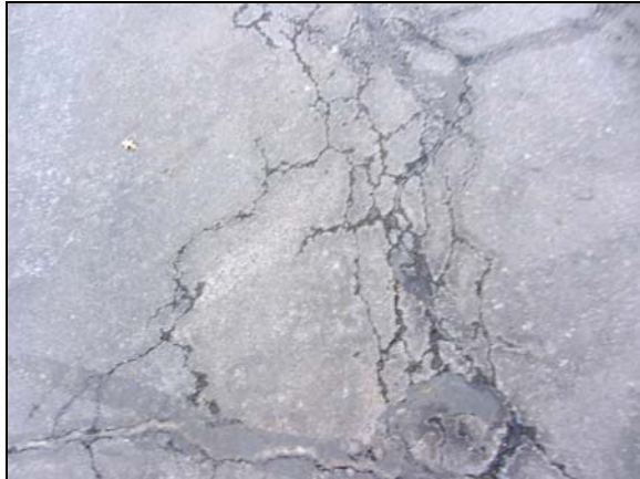
Photo #37. Alligatored asphalt pavement, Graystone Court.
