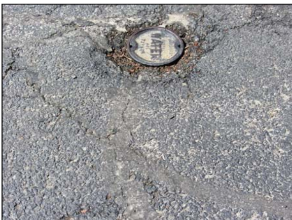
Photo #47. Typical failed pavement at utility access point.
