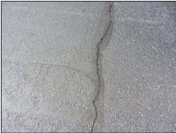
Photo #51. Typical open crack in asphalt pavement. Note failed crack seal.
