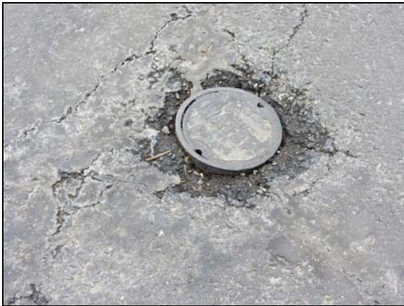
Photo #9. Failed pavement adjacent to utility access point, Granite Creek Lane
