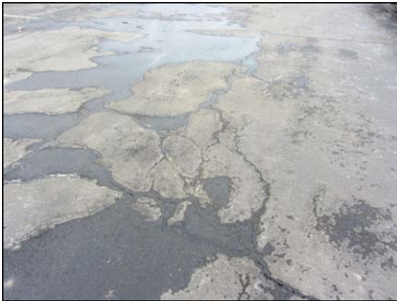
Photo #27. Alligatored asphalt pavement, Silverstone Court.
