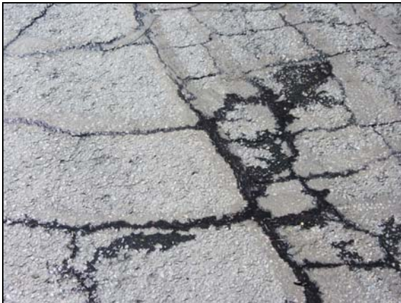
Photo #45. Alligatored asphalt pavement, Silverstone Court.
