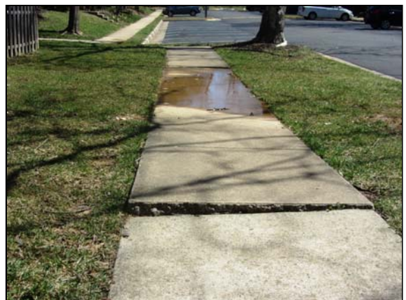
Photo #54. Displaced sidewalk is a trip hazard, typical.
