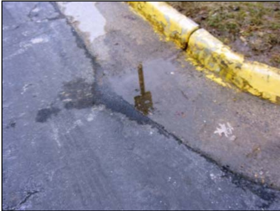
Photo #19. Typical depressed pavement and concrete curb & gutter may indicate damage to base materials and bearing soils beneath the asphalt pavement.
