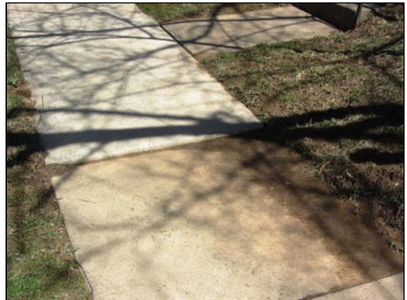
Photo #46. Defective grading and displaced sidewalk segments impound water and silt on the pavement, typical.
