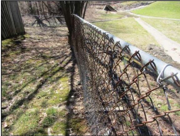
Photo #49. Rusty fence at stormwater impound facility.
