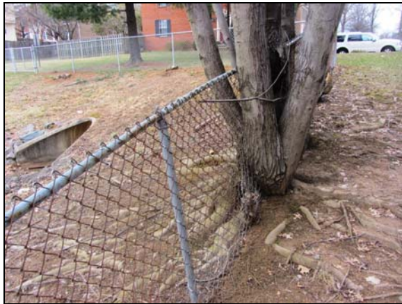
Photo #33. Stormwater fence is captured in the tree.
