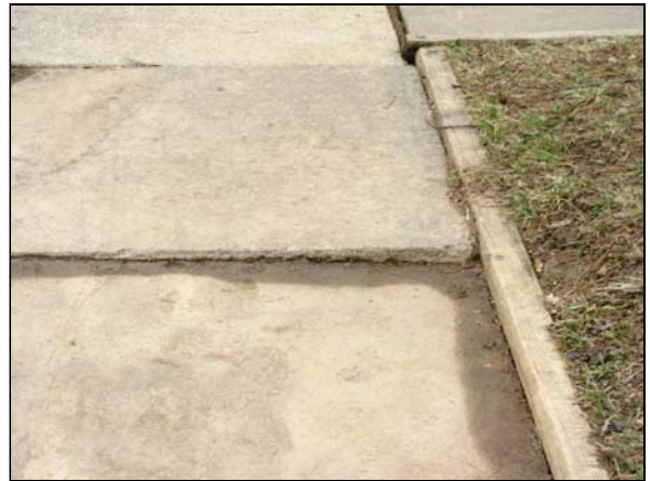
Photo #28. Displaced sidewalk, Silverstone Court.
