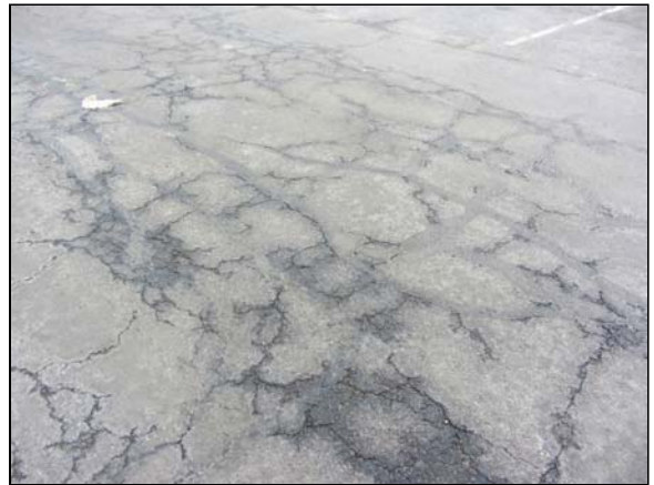
Photo #10. Severely alligatored asphalt pavement, Granite Creek Lane.
