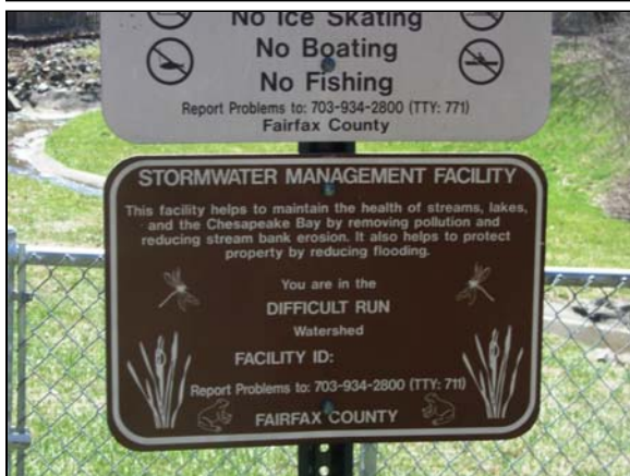
Photo #59. Stormwater impound does not have a "Facility ID".
