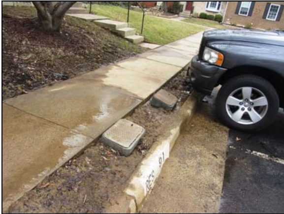
Photo #13. Defective grading between sidewalk and curb & gutter, Granite Creek Lane.
