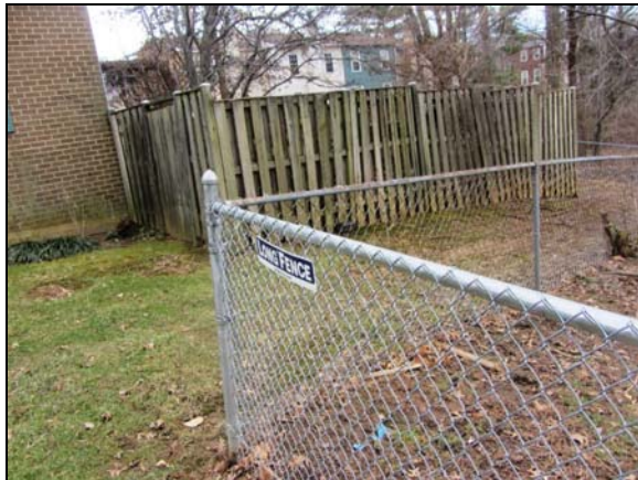
Photo #31. Fence around the stormwater impound facility. Note that fence in foreground has been recently installed and other fence sections are much older.
