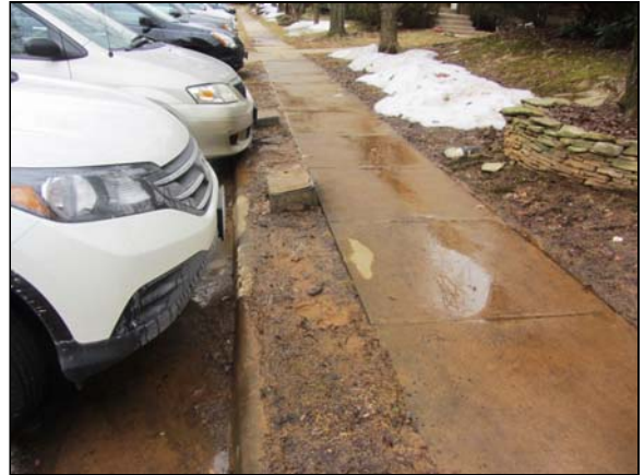
Photo #14. Improperly installed utility access points are potential trip hazards and may indicate that water services are not installed at the proper depth.
